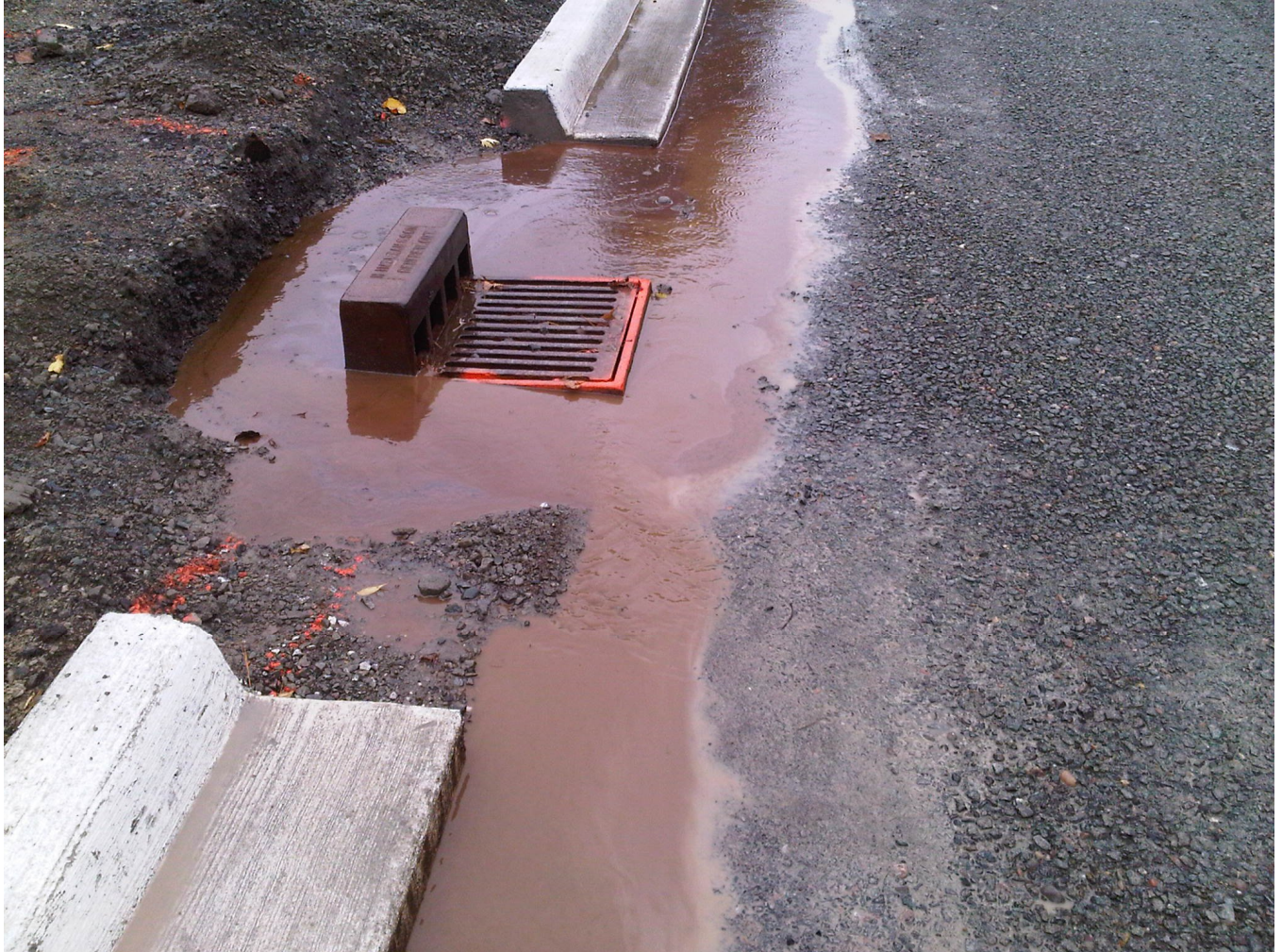
Contaminated water entering the storm sewer system
