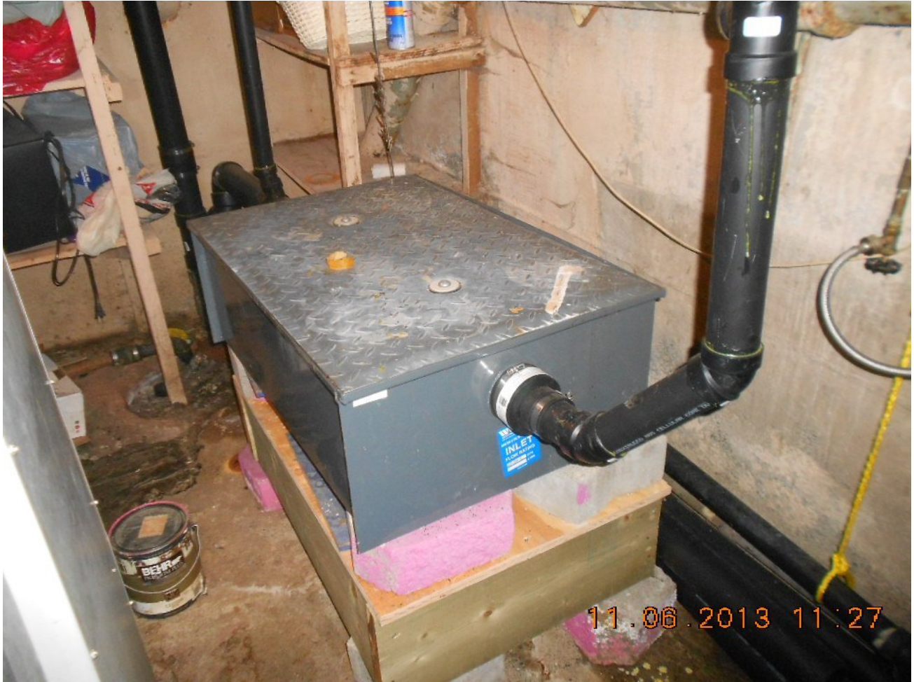
New grease interceptor installed
