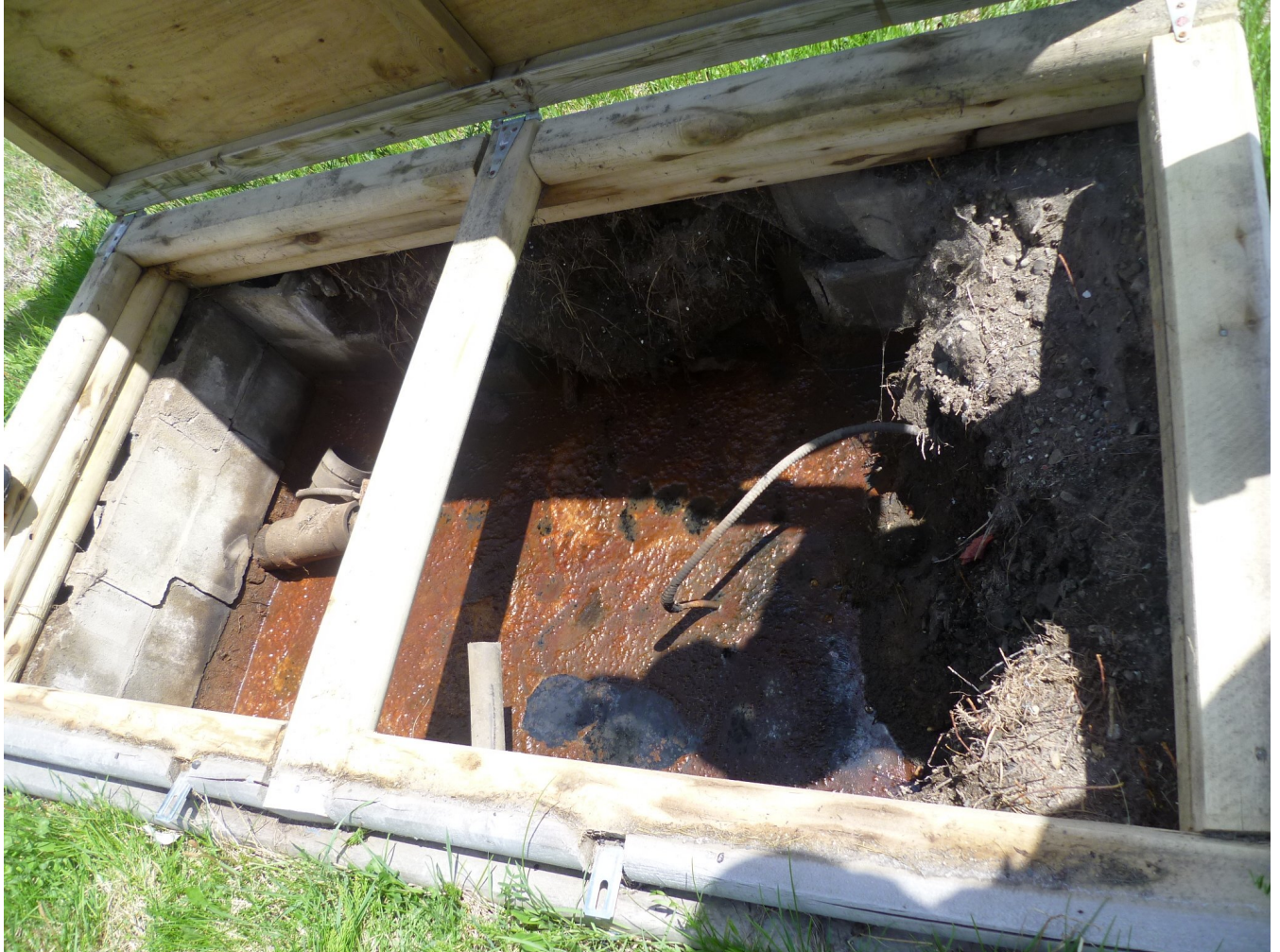
Damaged oil interceptor requiring repair / replacement
