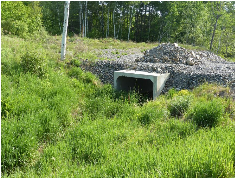
Photo 2: South Bay Road, Sudbury Culvert installed on Lots 63 & 64 on north side of South Bay Road File 701-6/21-01 Photography: June 3, 2021
