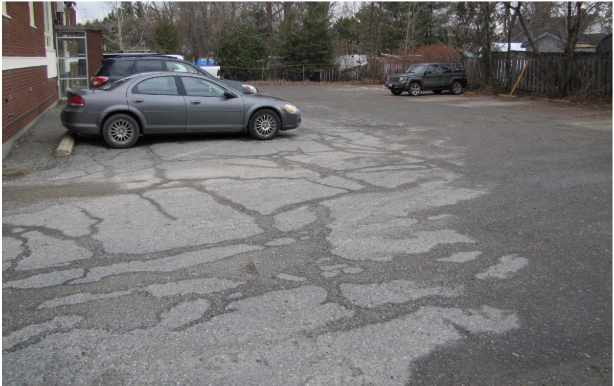
Photo 6. Parking area to the rear of the multiple dwelling across from the subject lands at 4 Poland Street. Photo taken looking south, on December 2, 2022. CGS file 751-6/22-17.
