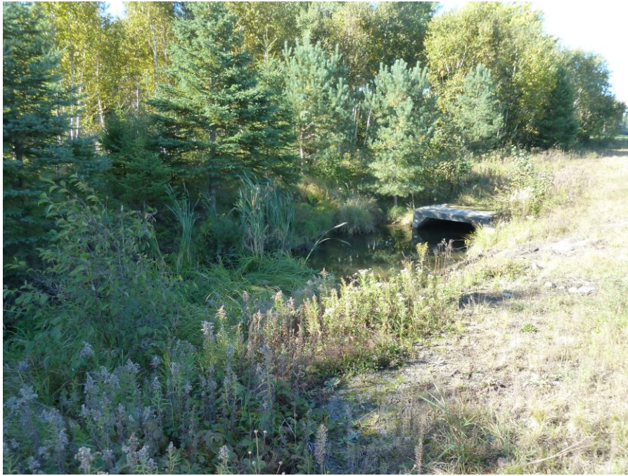
Photo 3: 0 Algonquin Road, Sudbury Drainage channel and box culvert on Algonquin Road File 751-6/22-009 Photography: September 29, 2022
