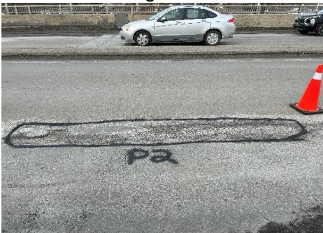
Prior to Patching
