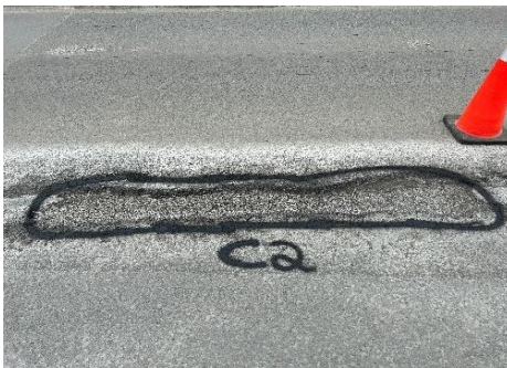
Prior to Patching
