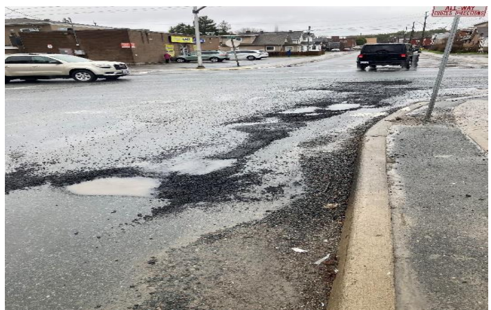
Figure 4b – Partial Failure of Patches
