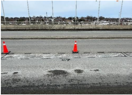
Prior to Patching
