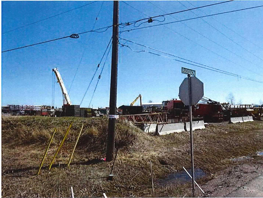
PHOTO 1 SUBJECT LANDS, 120 RADISSON AVENUE, VIEWED LOOKING NORTH EAST FROM THE CORNER OF MUNICIPAL ROAD 15 AND RADISSON AVENUE
