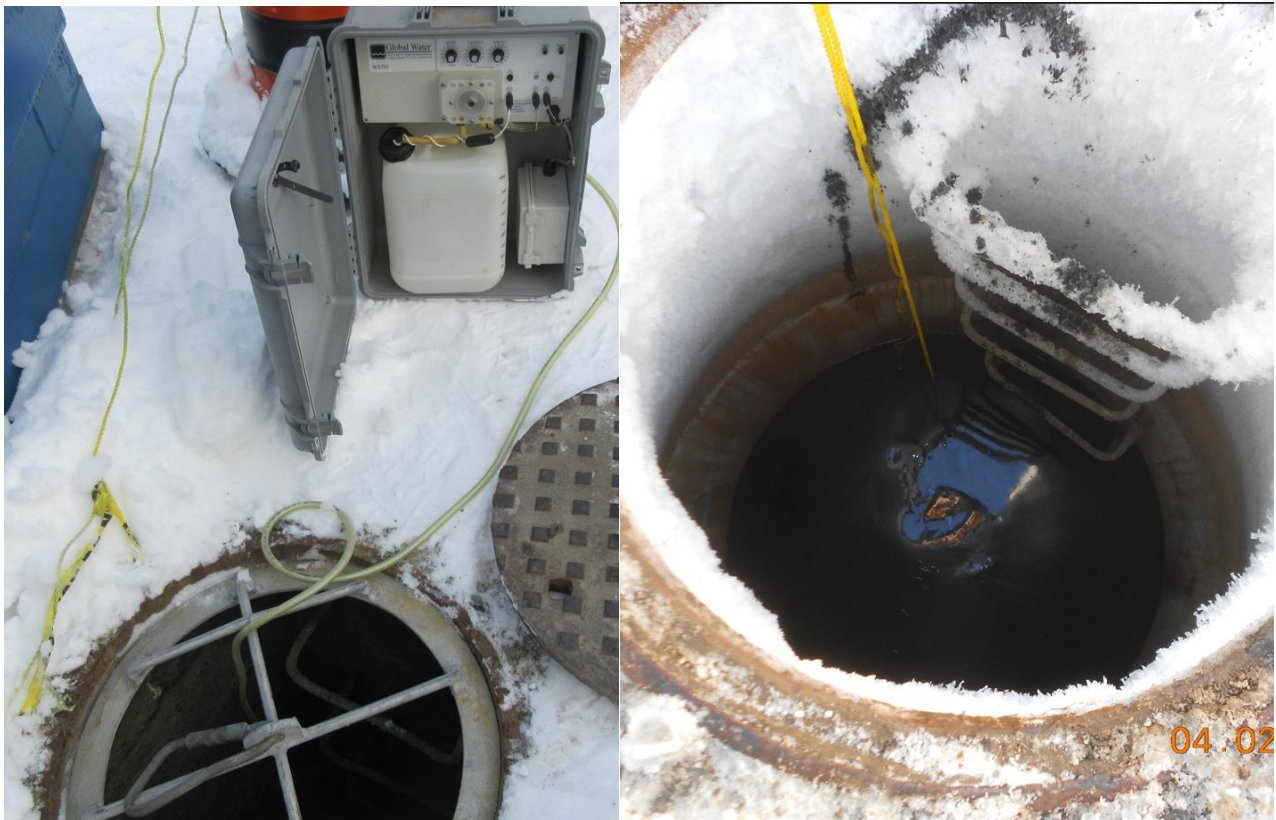
Test Maintenance Hole with Sampling Equipment (left) and Waste Motor Oil Found in Maintenance Hole (right)
