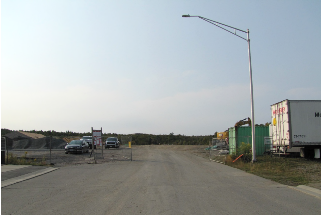
Photo 1. Subject lands at the end of Billiard's Way, facing south, with construction of Billiard's Green row dwelling units on the left and Highway 17 in the distance. Photo taken September 12, 2024. CGS File 751-6/24-14.
