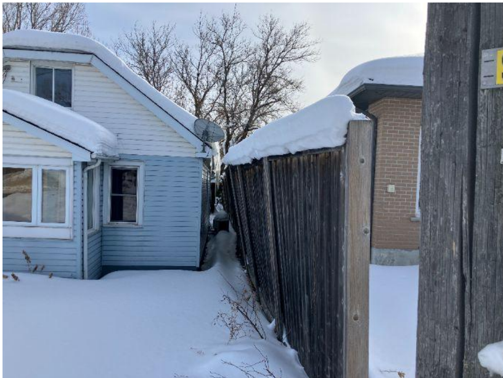
Figure 2: Wood fence between subject property and abutting medical clinic to the west (February 12, 2026)
