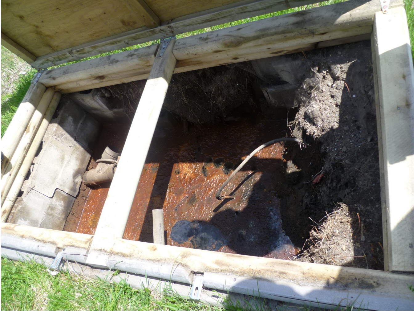
Damaged oil interceptor requiring repair / replacement
