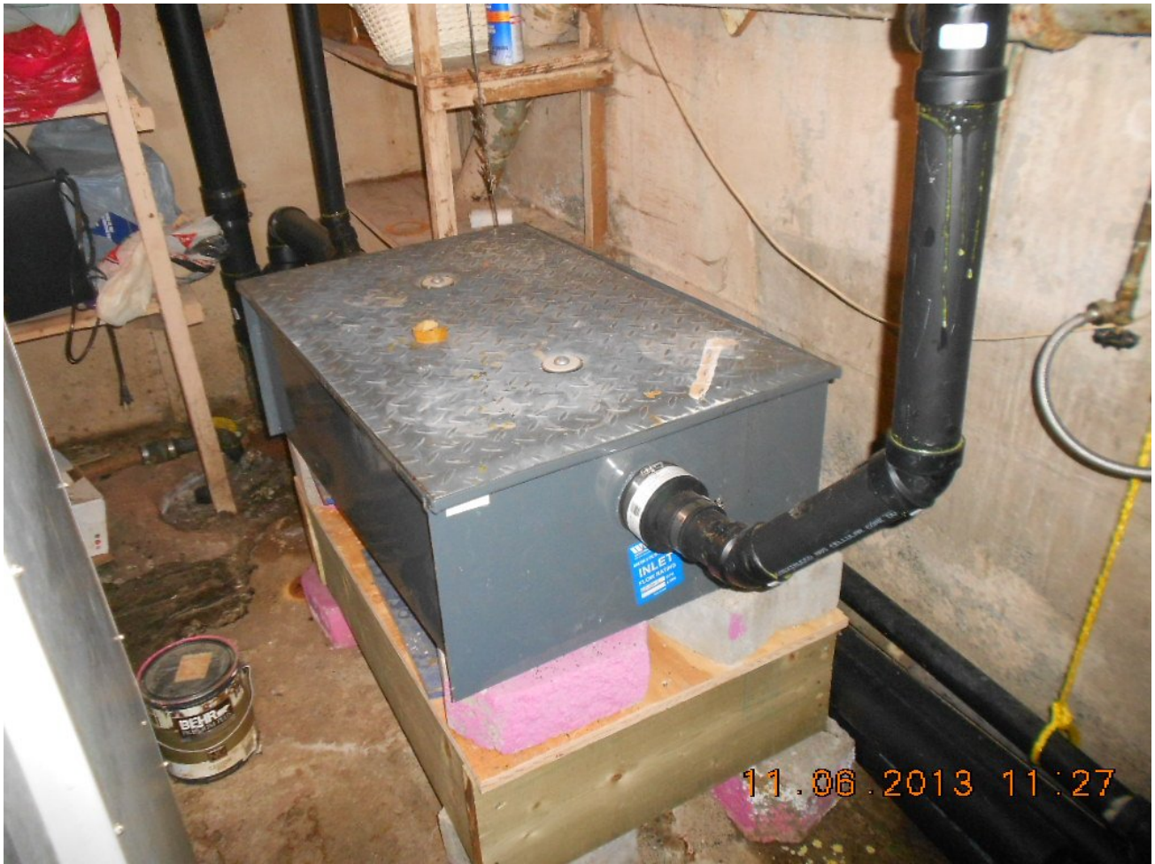
New grease interceptor installed
