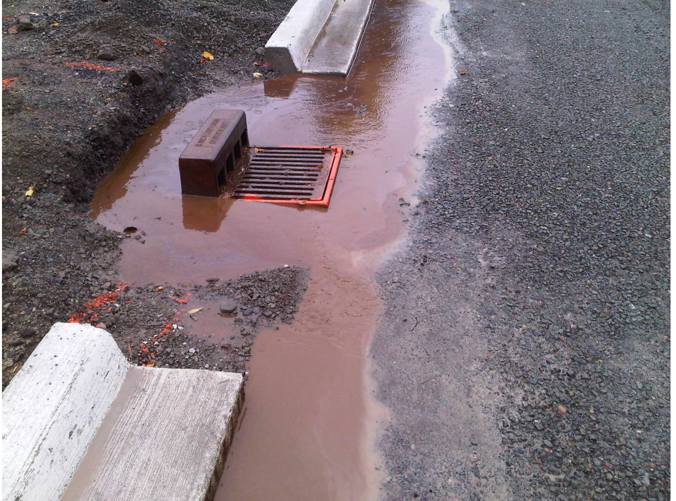
Contaminated water entering the storm sewer system
