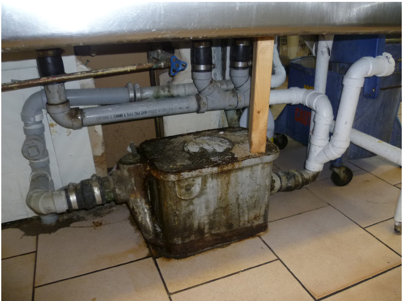
Old grease interceptor requires replacement
