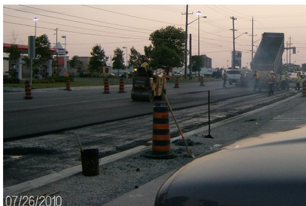
Exhibit 1 – Inferior Asphalt Supplied
