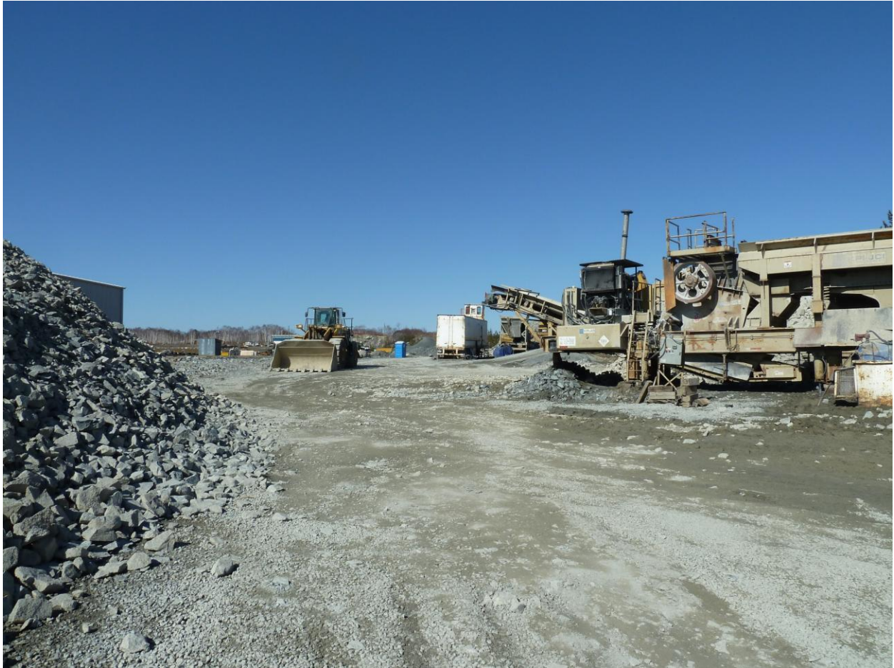
Photo 3: 234 Fielding Road, Lively Site alteration and heavy equipment on PIN 73372-0232 (Rintala Construction) File 751-8/20-2 Photography April 11, 2020
